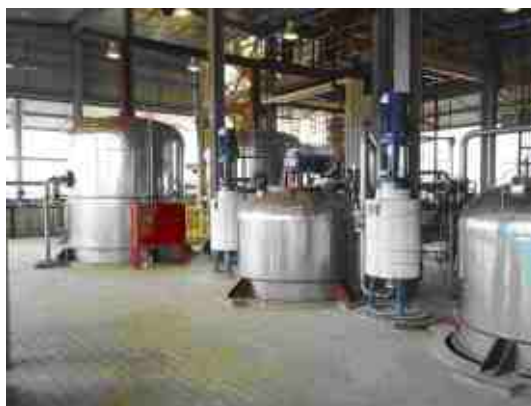
Oil Refining Equipment
