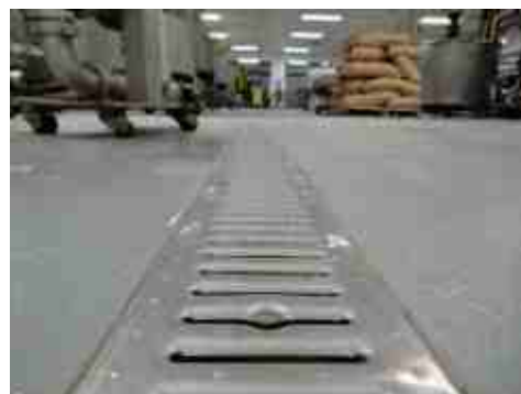
Covered drains inside the premises to avoid any water logging
