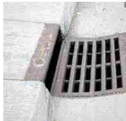
Cover all the drain holes in the premises with grill
