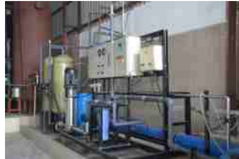
RO system for potable water
